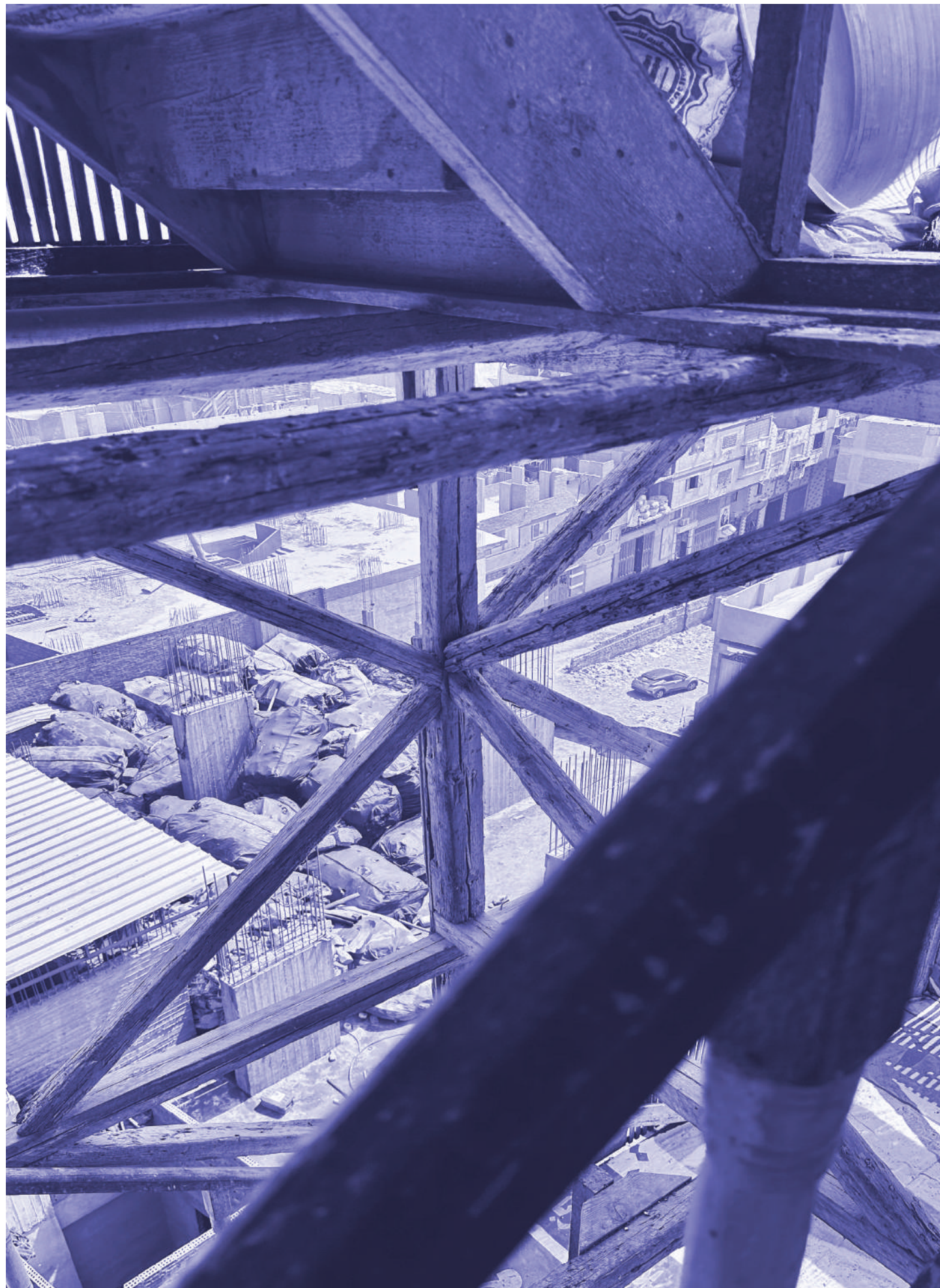
Fig.4 – View from the first floor of the “Koka” pigeon tower. Copyright to the author.
