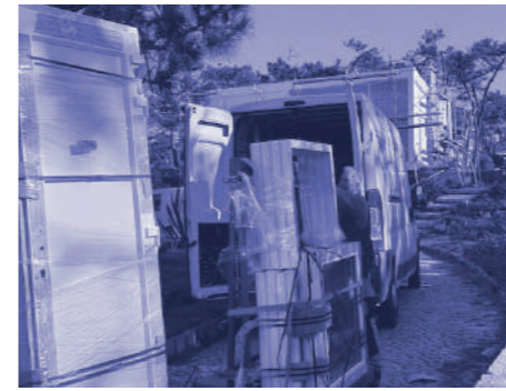
Fig.4 - PVC window frames awaiting installation at the same house, November 2025. The profile thickness exceeds the original hardwood frames — specified by the architect at 1:10 detail — by a factor of three. The intervention was undertaken without a building permit. Source: author, 2025.
