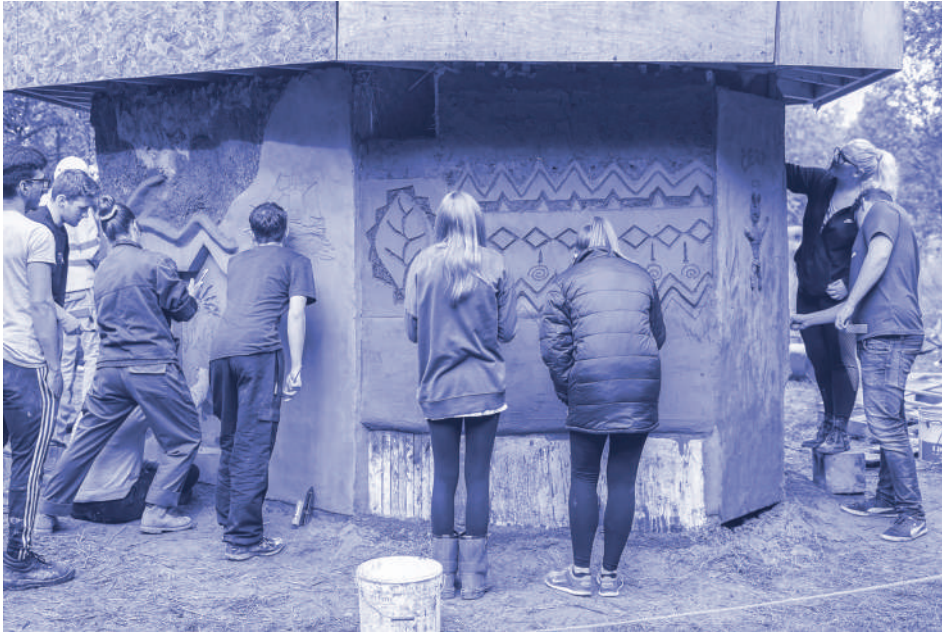
Fig. 2 Construction of Lincoln Hexagonium: each builder makes their own mark. This is what makes this building unique and what is a unique value of low-tech
