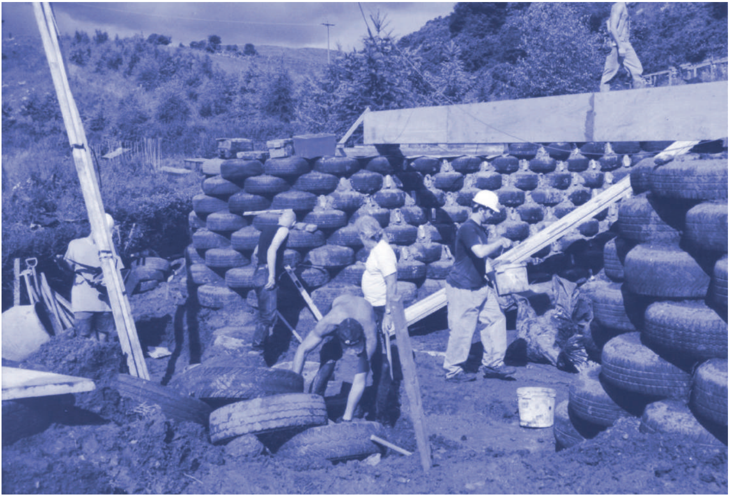
Figure 8. Earthship construction by Michael Reynolds, who like other low-tech architects developed a cheap construction for poorer parts of the society
