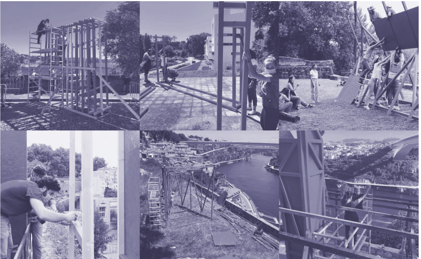
Fig. 9 - Work in progress construction weeks of all teams. Follies 1 to 6, from top left to bottom right.
